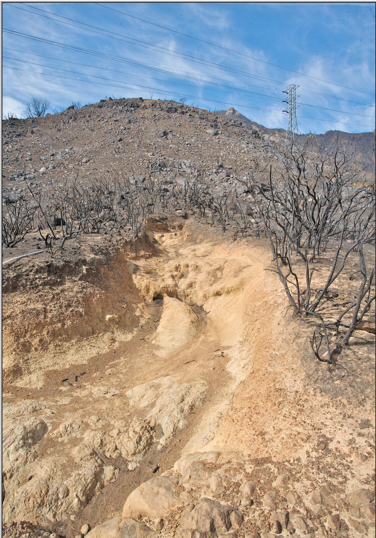
One picture often says it all. By burning away the vegetation the Jesusita Fire of 2009 exposed what poor trail design, lack of maintenance and improper erosion control techniques can do to a trail over time.
