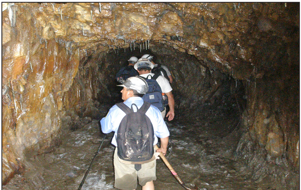
Once a year city water inspectors walk through the tunnel to check for damage to the ceiling and walls. The tunnel is four miles long and in places less than five feet high. Considering the tunnel was built a century ago, it is in amazingly good condition.
